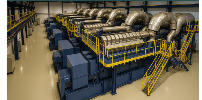
Primary and Backup Power for Data Centre
